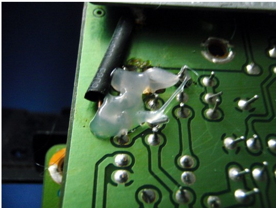
Above: Hot melt glue thinly applied to the PCB and new tracks.
